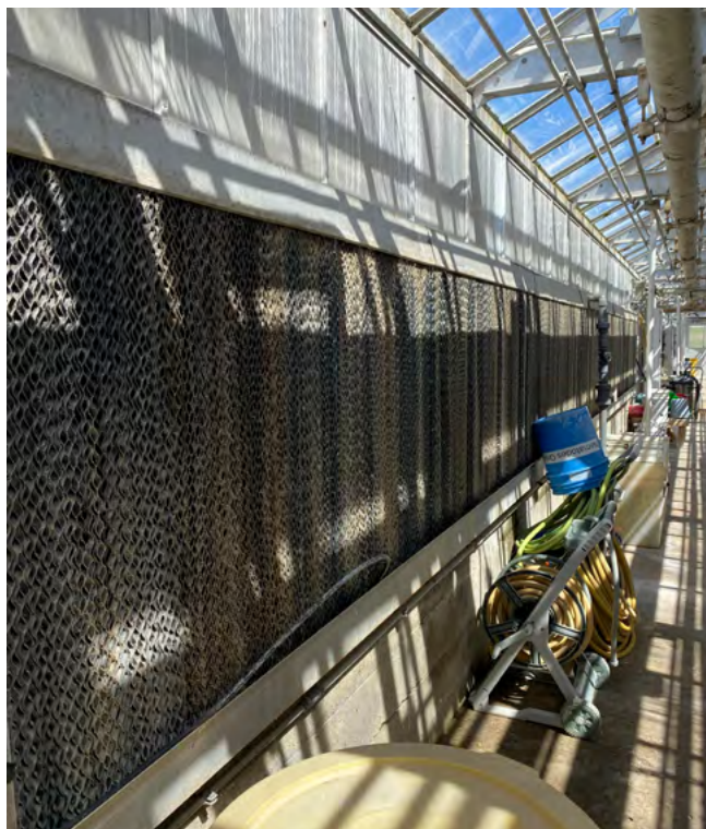
Evaporative cooling system. Photo: Andrew Demetri
